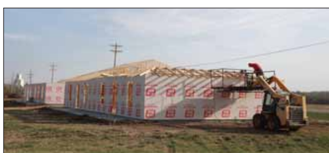
Work on new houses moves forward Tuesday morning on the southern edge of Ellsworth.
