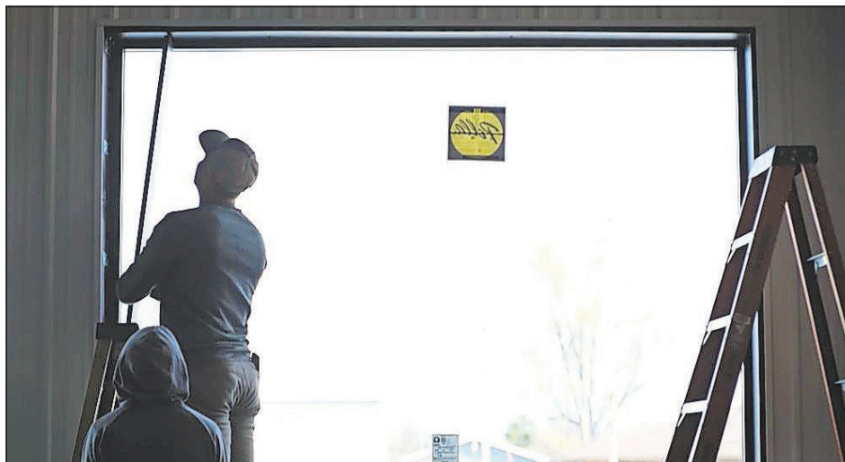
Casey Venters and his son measure wood used in the window frames of the store being built in Dighton. CALEN MOORE/KNS
