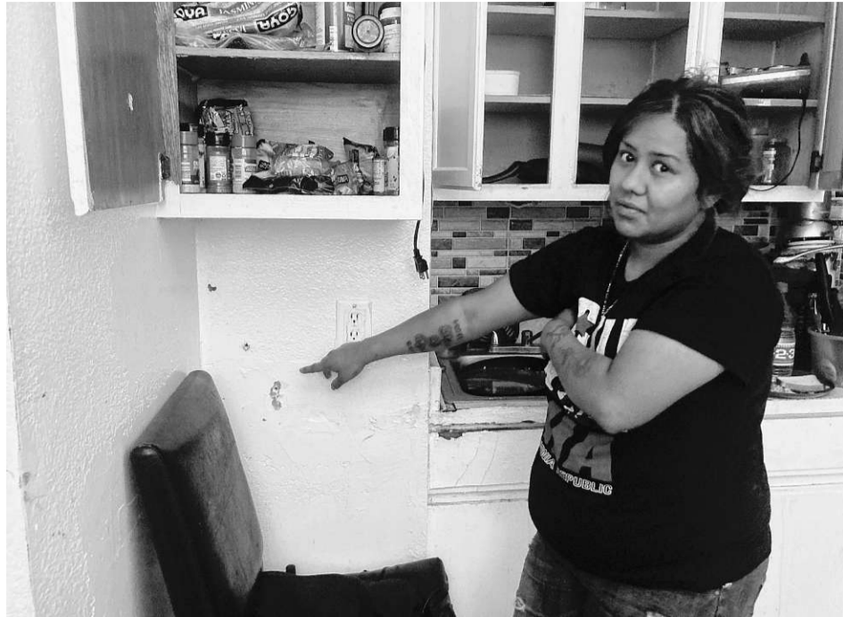
Elizabeth Ojeda, 33, points to the holes in her kitchen wall left by three bullets that flew in from the apartment across the hall, allegedly fired by her friend and neighbor, Brayon Noe Arguijo-Mejia, 20.
